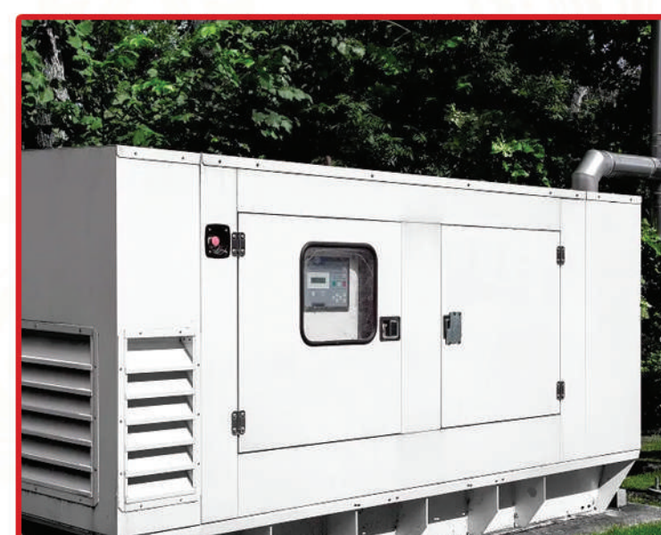
COMMON AREA POWER BACKUP
